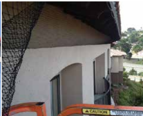
StealthNet installed under eaves prevents swallows from building mud nests.
