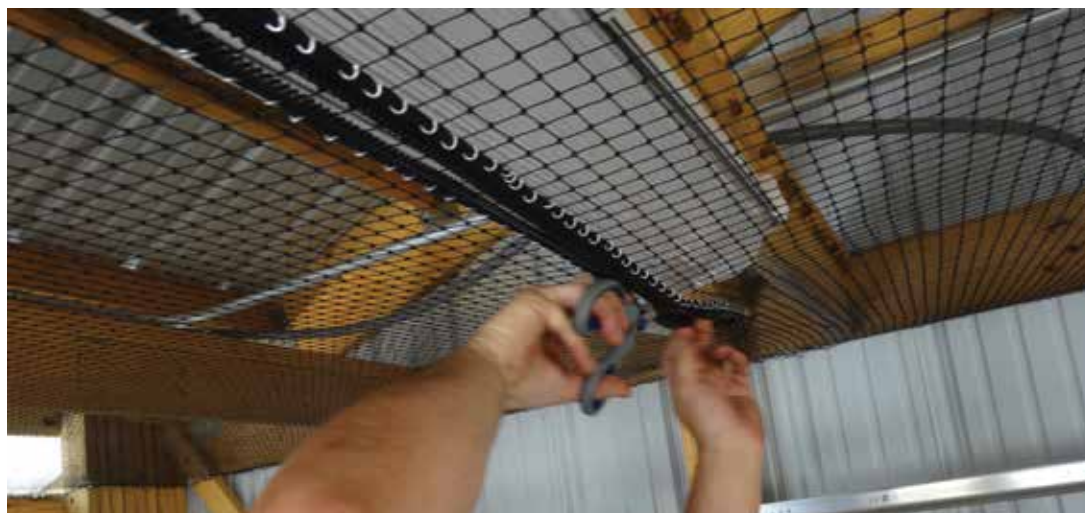
StealthNet installed underneath pipes and beams in a newly constructed barn keeps all birds out. The zipper being installed allows access to the lights.
