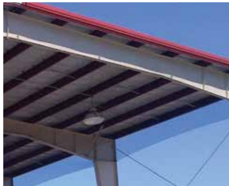
Netting installed 18 in. under this hangar completely excludes birds from the structure.
