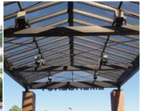
Vehicles parked under this hospital portico no longer suffer damage from bird droppings.
